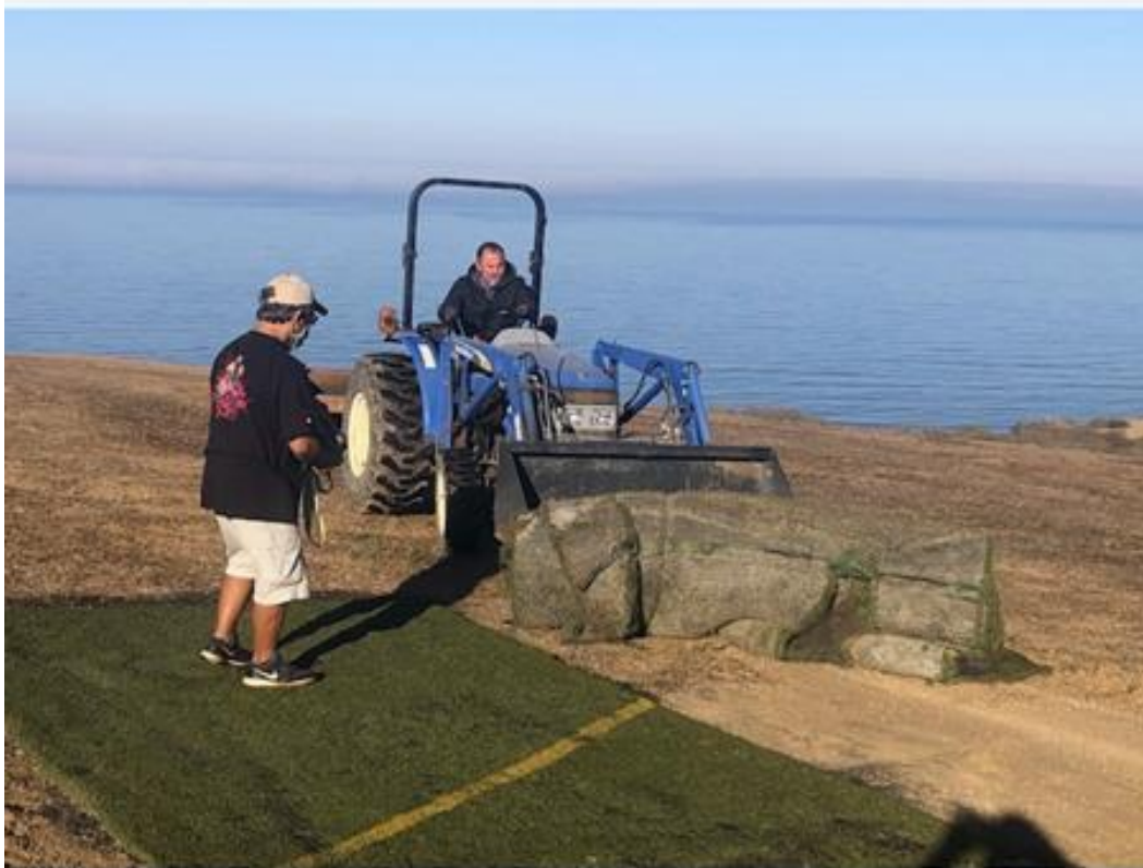
Halloween Day: Our last install day of doubling the width of the landing strip. The two workhorses throughout the whole project; Ray and Carlos. Thanks guys! (Mark Baldacchino photo)
