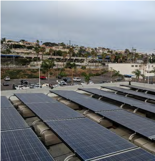
Just a few of the rooftop solar panels (Dale Gottdank photo)
