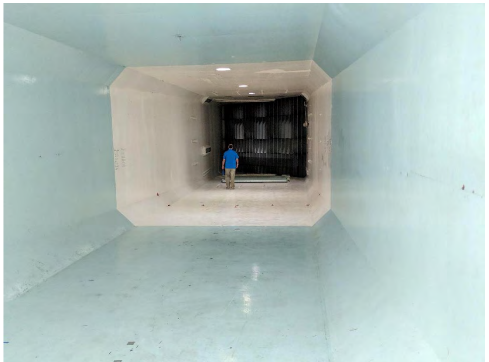
The chamber is much wider at the far (exit) end than at the honeycomb, as evidenced by Marty standing in front of each. (Dale Gottdank photo)
