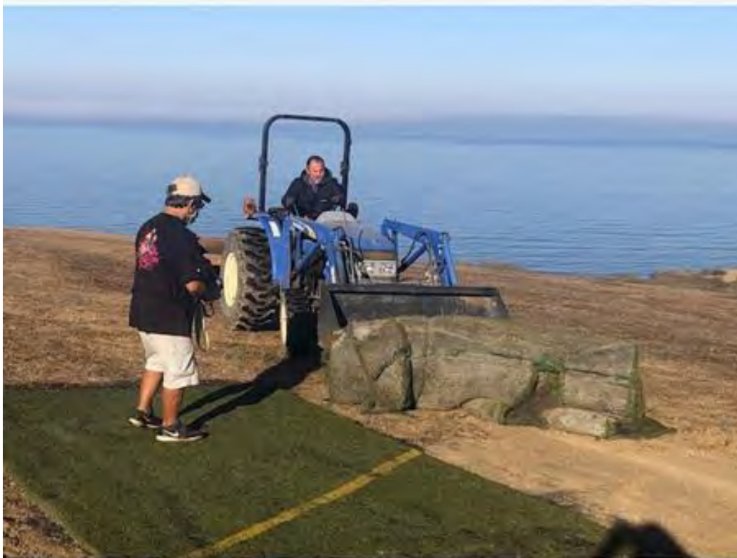
Halloween Day: Our last install day of doubling the width of the landing strip. The two workhorses throughout the whole project; Ray and Carlos. Thanks guys! (Mark Baldacchino photo)
